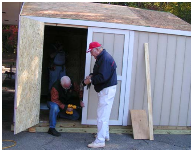
Jerry Colclasure and Earl Cosgrove putting the finishing touches on the MG shed.
