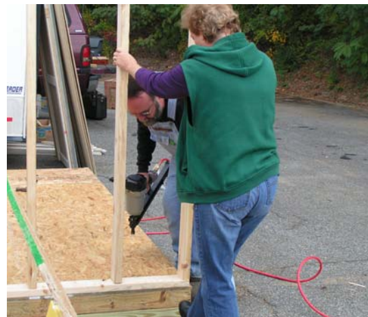
Marsha Rauscher puts her foot into it while John Shipley nails the flooring.
