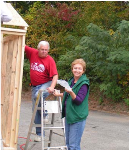
Don and Marsha Rauscher help to secure the new siding on the new storage building.
